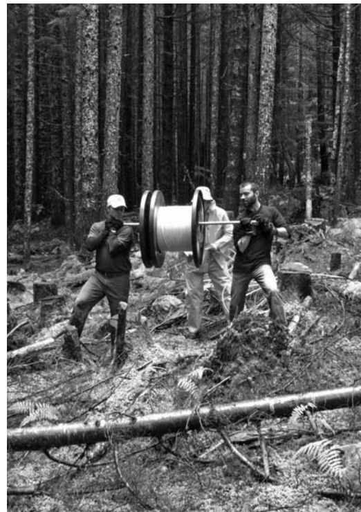
Figure 8. Installing the fiber-optic cable through a gap treatment. Photo: J. A. Lutz.
