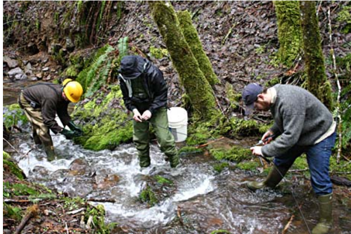
Figure 2. Laying a fiber-optic cable in the HJ Andrews experimental forest in Oregon in the spring of 2007
